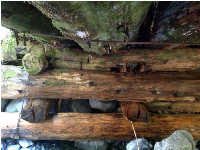
left abutment top crib log cracking vertically and horizontally
